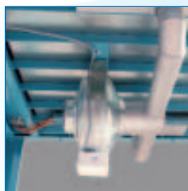
Ventilator for air supply
